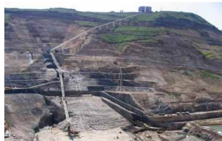
Figure 5.4.1.1: A conveyor system transports RCC from the top of a mountain to the dam site
