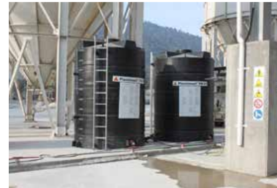
Figure 2.4.1: Sika® Plastiment® storage tanks
