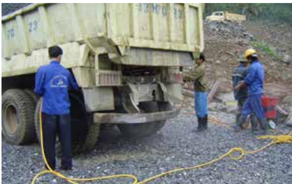
Figure 5.4.2.2: Workers wash a haul truck's tyres to prevent contamination of lift surfaces
