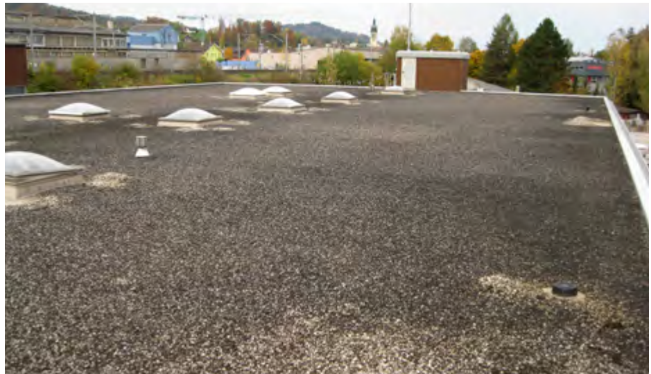
Fig. 4: Overall view of the roof of the Brunner Building in Flawil (Switzerland)
