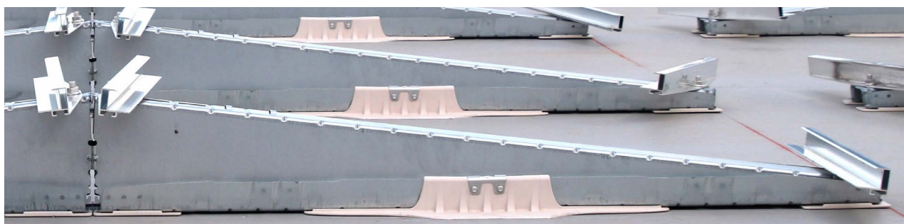
SSM2 mounts with SarnaRoof® Clicks, pads, metal bracket securements and short rails for the east-west installation
