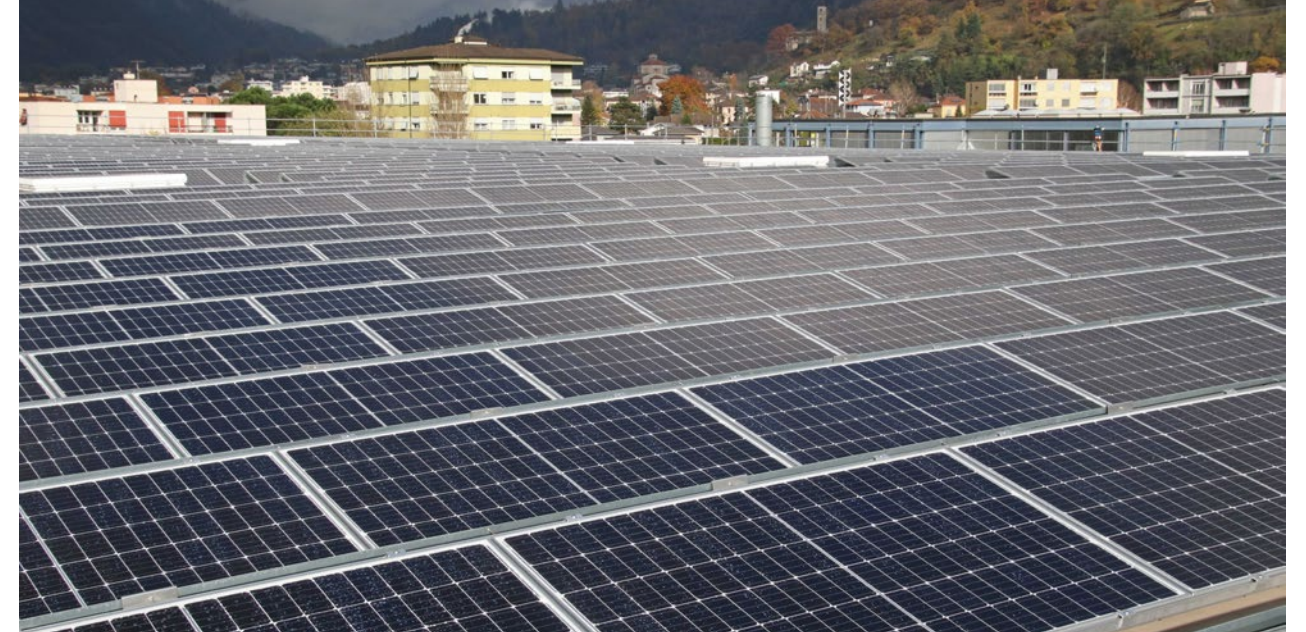
Photovoltaic plant, Raiffeisen BiascArena, Biasca, Switzerland.
