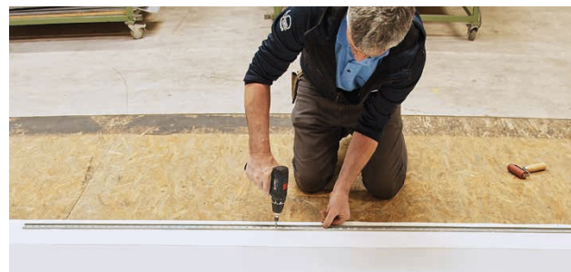
2. Installation of Sarnabar® fastening profile with Sarnafast® Fasteners and Sarnafil® T Welding Cord.
