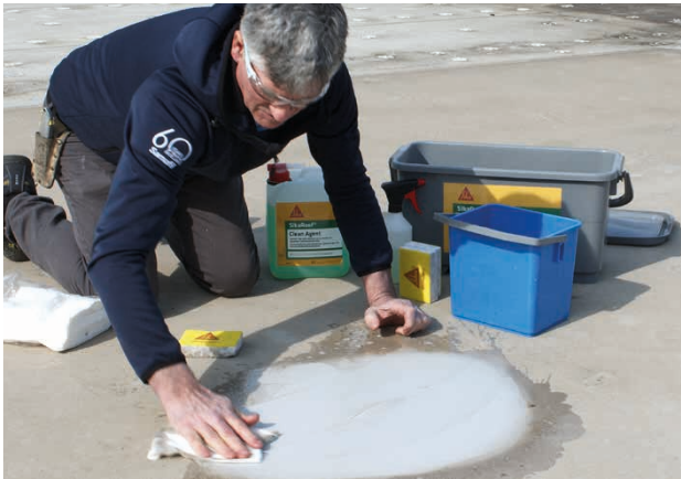
5. Proper cleaning of existing area to be repaired (as explained under CLEANING).
