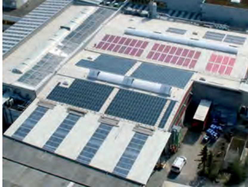
2008 | Solar park Stuttgart was opened to display various solar technologies
